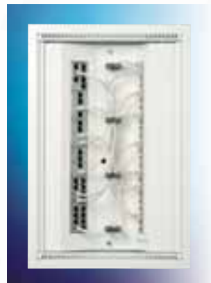
11. Place the patch leads neatly in the middle of the distribution cabinet with the help of guides provided.
