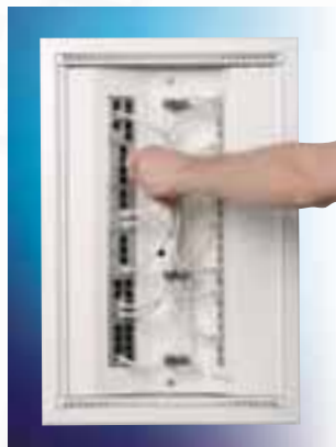
10. Connect patch leads between the patch frame and the TV amplifier, telephone and data modules.
