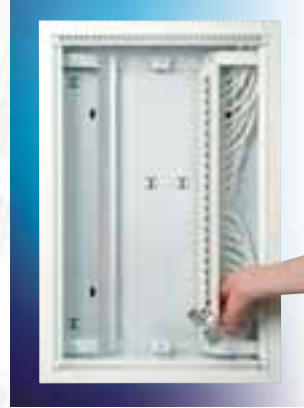
3. Insert the terminated RJ45 connection jacks into the ports of the patch frame, and keep track of the numbers (1-26) as marked on the patch frame.
