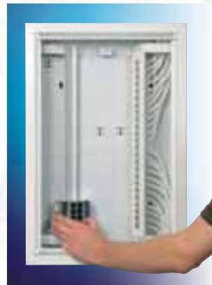
7. Install the active modules (telephone, data and TV amplifier) on the DIN rail provided in the distribution cabinet.
