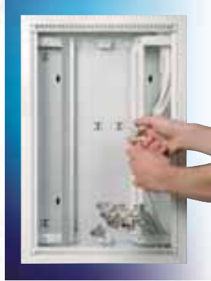
2. Terminate all the installation cables with RJ45 modular connection jacks in accordance with the procedure as described on page 16.
